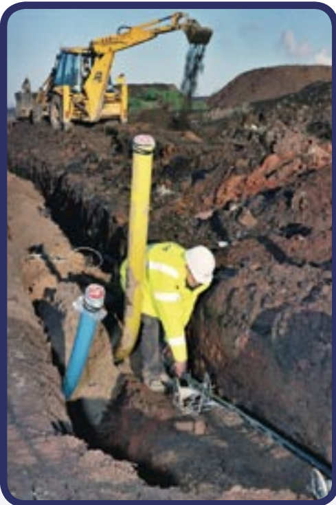
Core offer complete infrastructure solutions
