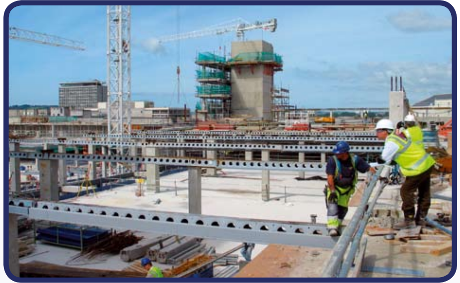
BRC Deltabeam Structural Construction System at the Drake Circus Project in Plymouth
